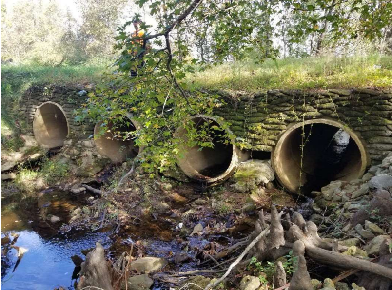
Culvert outlet shows that the culvert is perched
